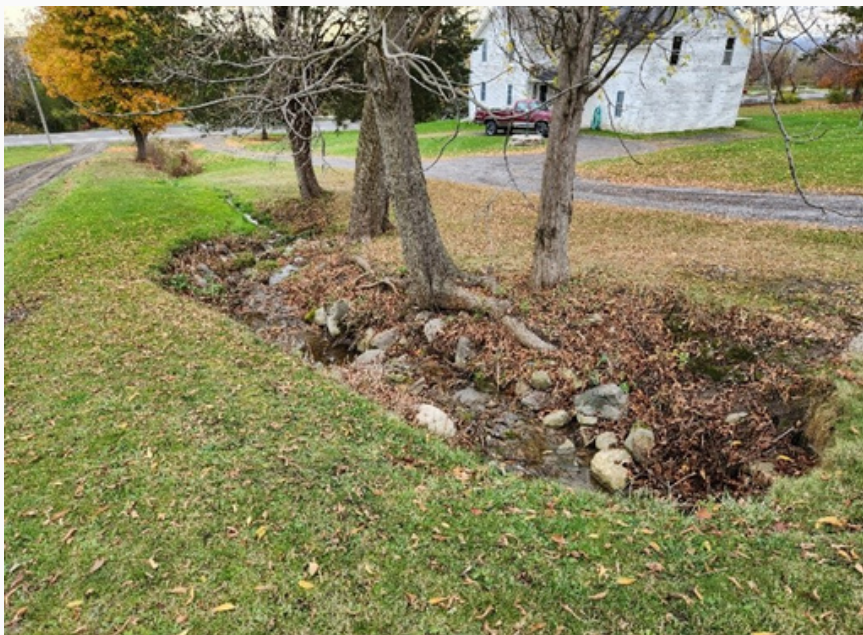
Figure 3: Phase II of the ditch project is scheduled for completion in 2024. Note how erosion is cutting away at the bank.
